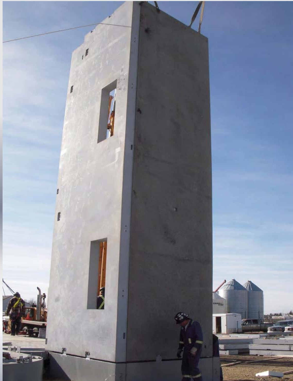
First corner has to be secured from a 100 km./hr. wind blowing without notice. At 60 km./hr. operation stops for safety. However, with rain and/or snow the operation continues.
