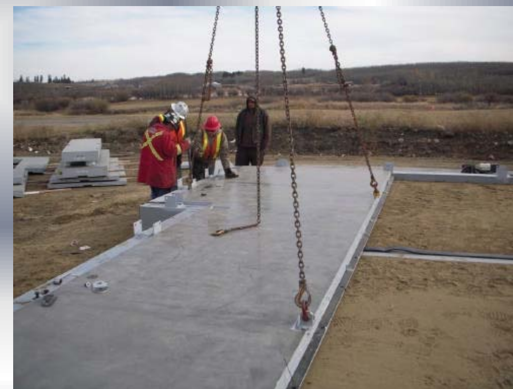
This picture shows the installers for the first time trying to utilize what they learnt on site with respect to levelling and plumbing; prior to tightening the bolts and moving forward to the next panel. A very fast learning curve to installers totally unmatched by any other system of this scale.
