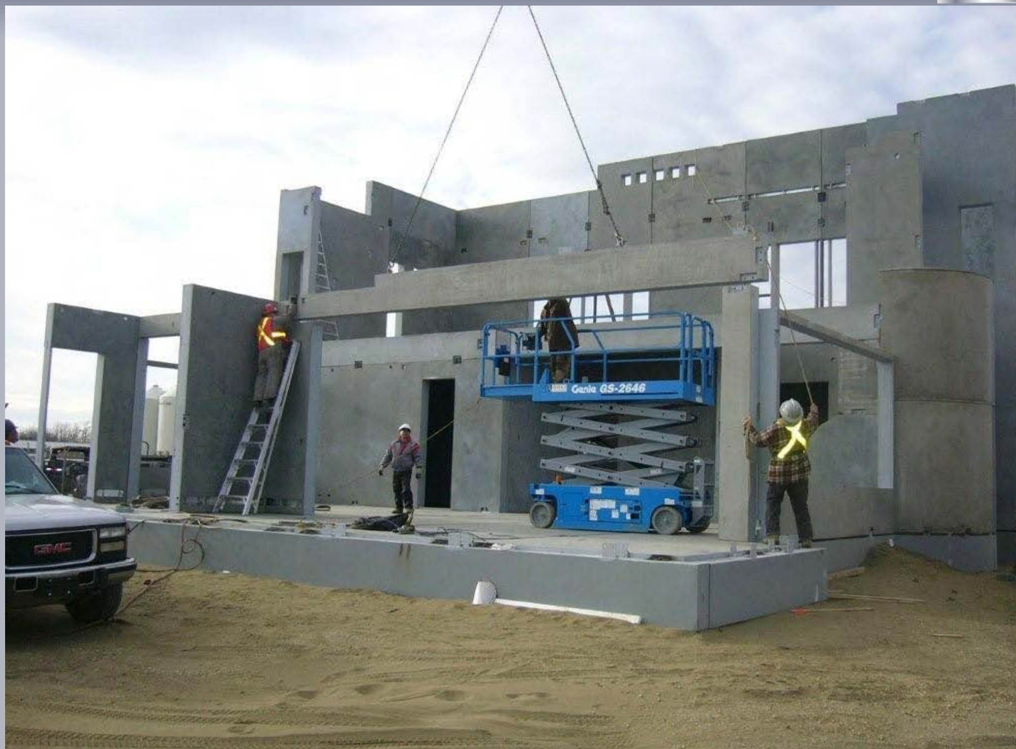
Assembly of the second IHI beam above the display area of the HCD Technology Center. Same comments as before.
