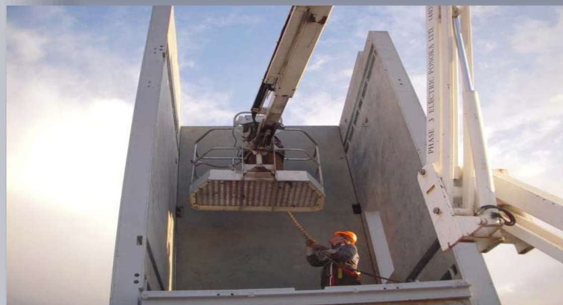
Tack-welding bolts after levelling & squaring all corners by the welder in the man lift.
