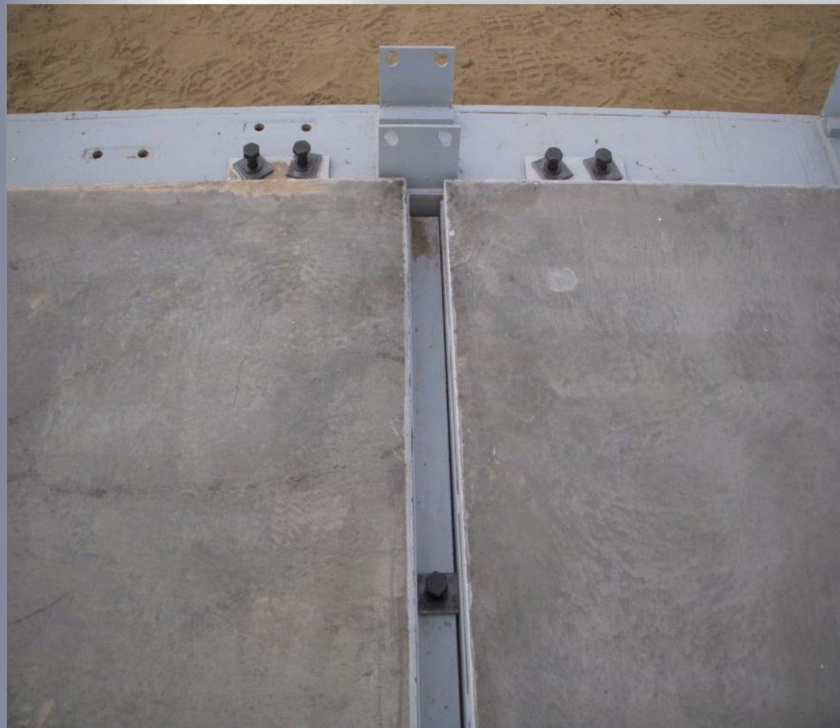
This picture shows again a perfect fit. Bolts are not tightened prior to levelling and plumbing.
