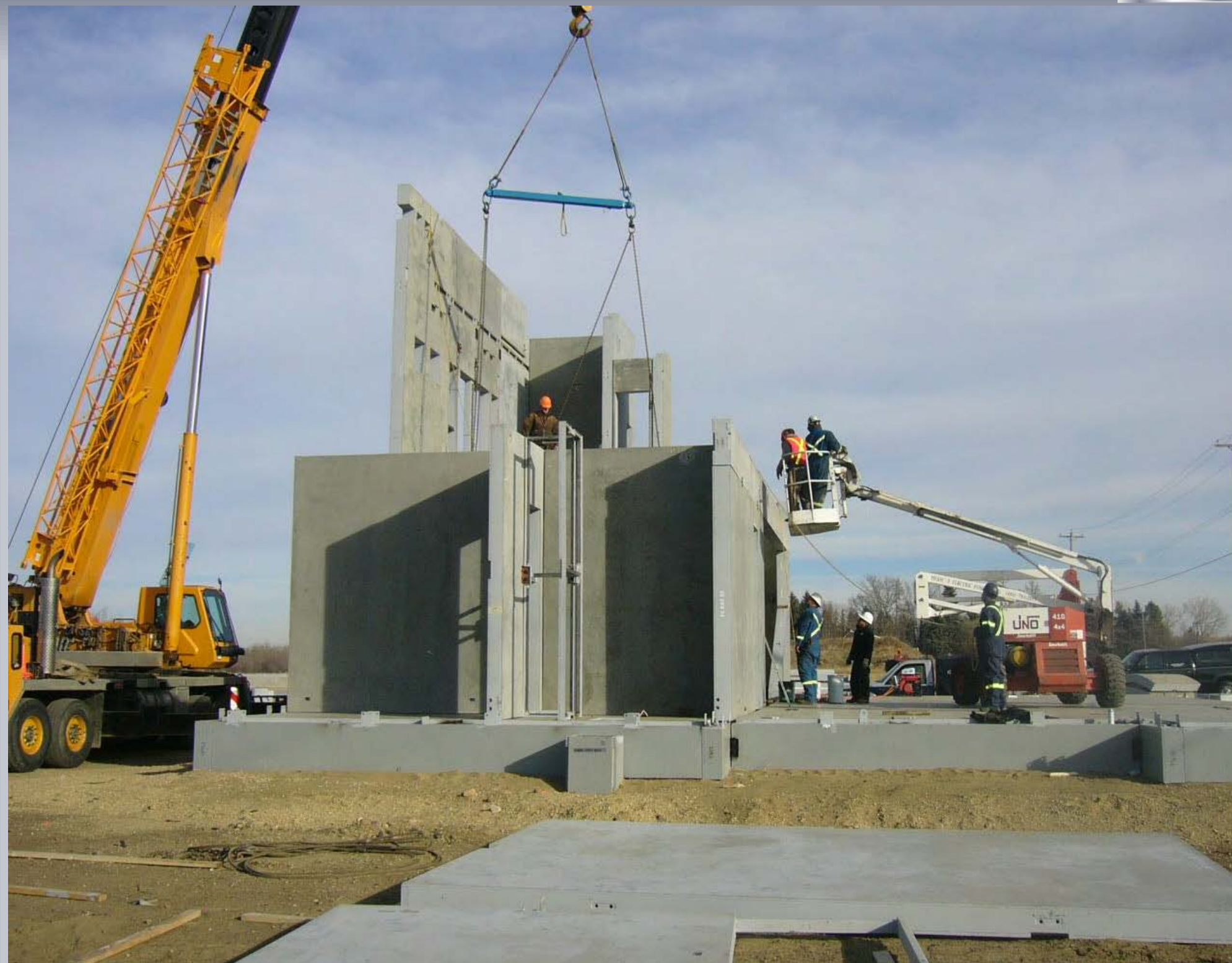
View from the South side of the property showing the installation of one of the second floor slabs.
