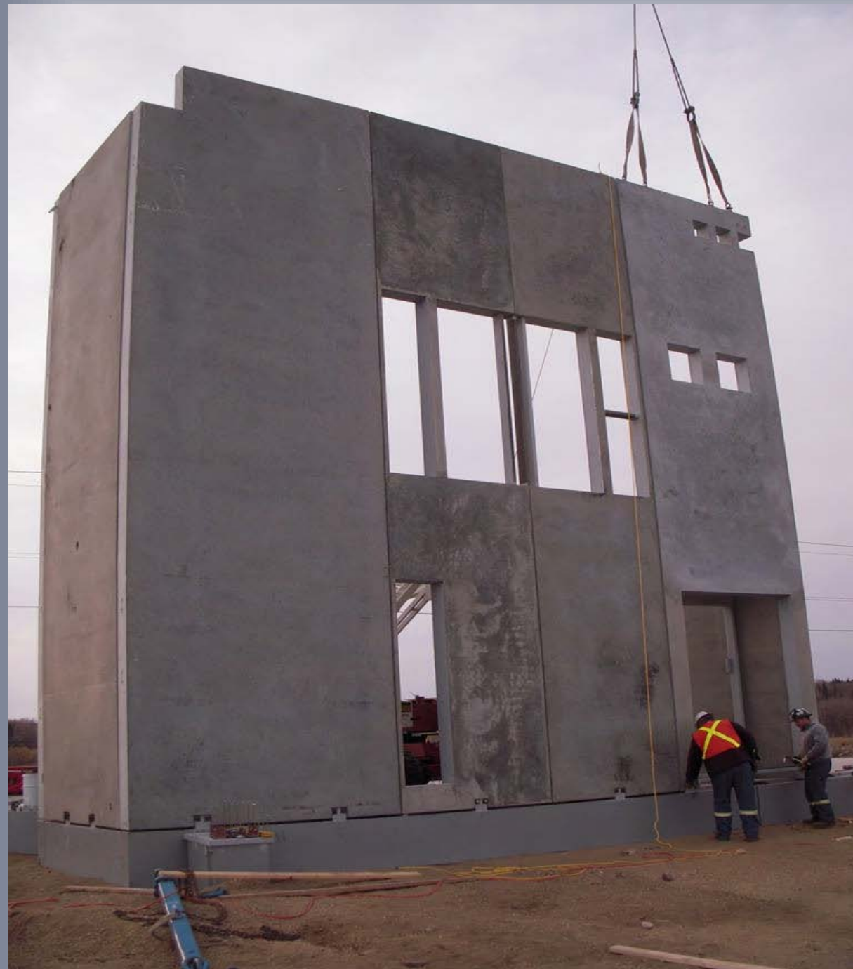
The alignment and the smoothness of the 12,000 psi high-strength concrete is very visible.
