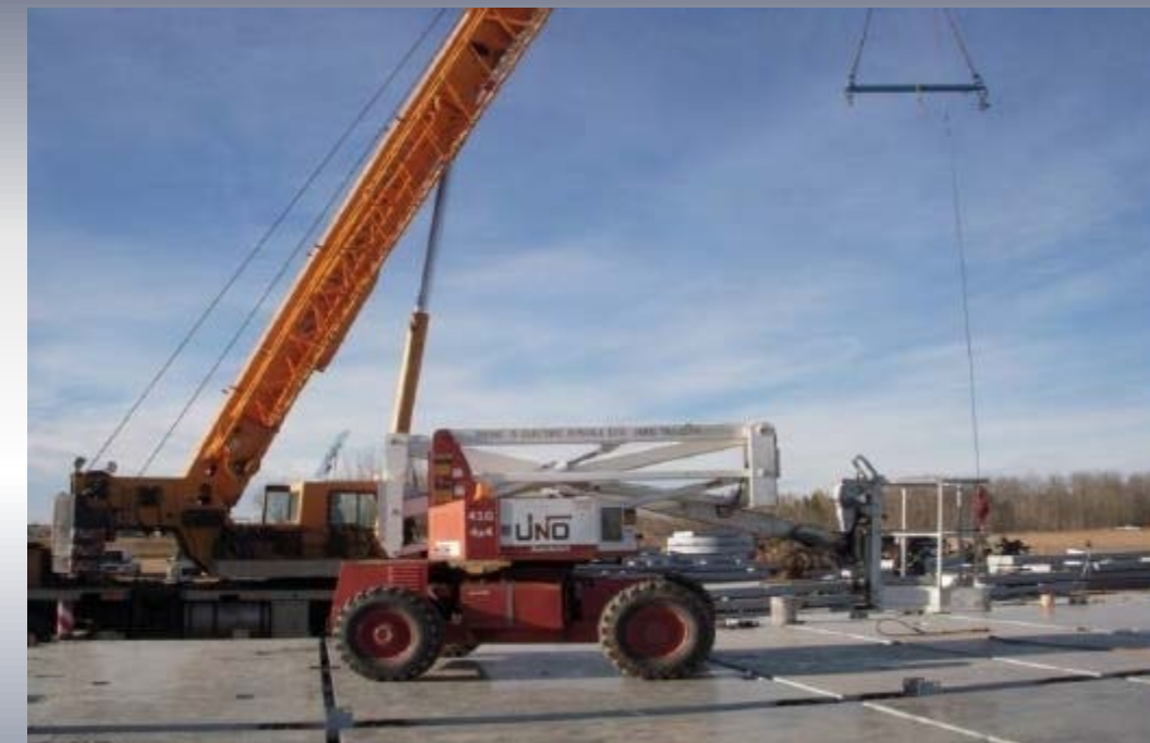
We had to lift the man lift on the panels, since the surrounding soil was not levelled and too windy to operate in a stable manner. The machine weighs 6 tons and the average thickness of concrete is 2.5 cm. Certainly above is not achievable by any other system.
