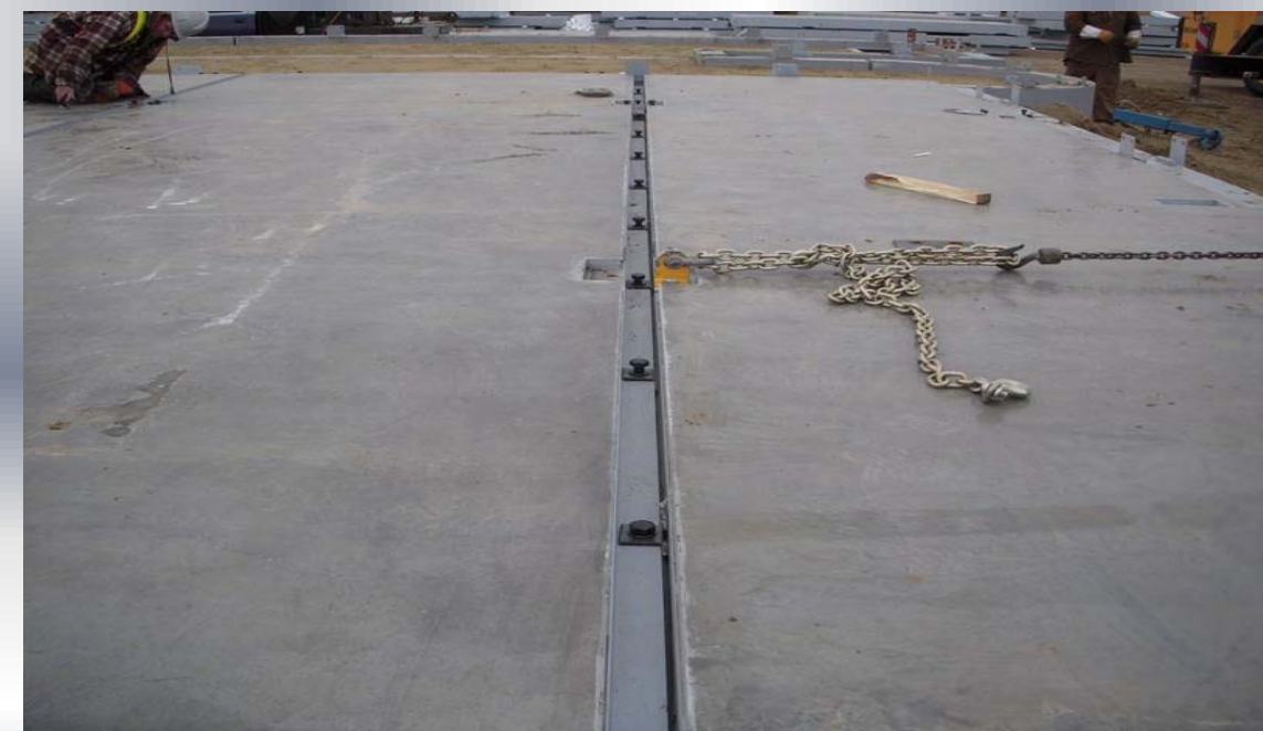
All bolts are perfectly lined up after tightening the IHI slab to the beam foundation using a 1.5 ton pulling device. Though the panels are extremely strong, they can be easily worked around for perfect alignment unlike any pre-cast or conventional cast-in-situ.
